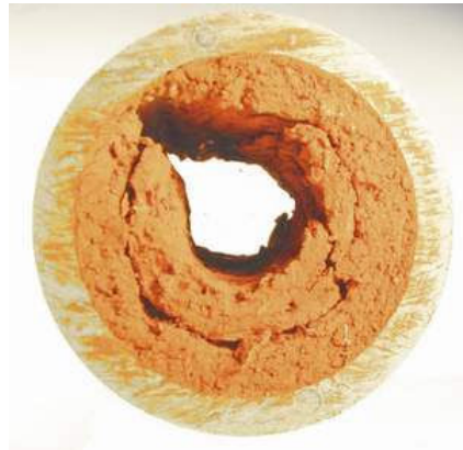
Fig. 5: Blocked waste water pipe after high pressure cleaning behind the polisher
